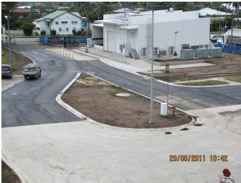
Nebo Road WTP - New Switchroom & Chemical Dosing Building, roadways and storage shed
