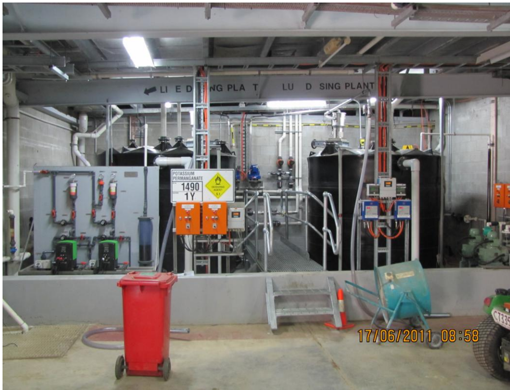
Nebo Road WTP - New Potassium Permanganate Tanks, Dosing Equipment installation nearing completion
