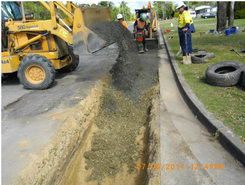
South Mackay Trunk Main - Backfilling and road reinstatement after laying of pipe along Main Street Bakers Creek
