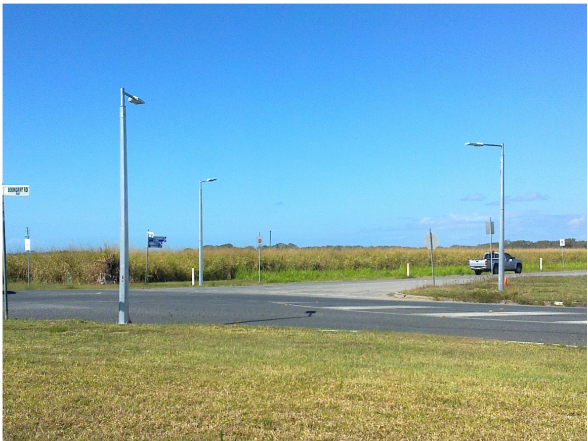
Milton Street / Boundary Road Intersection Street Lighting
