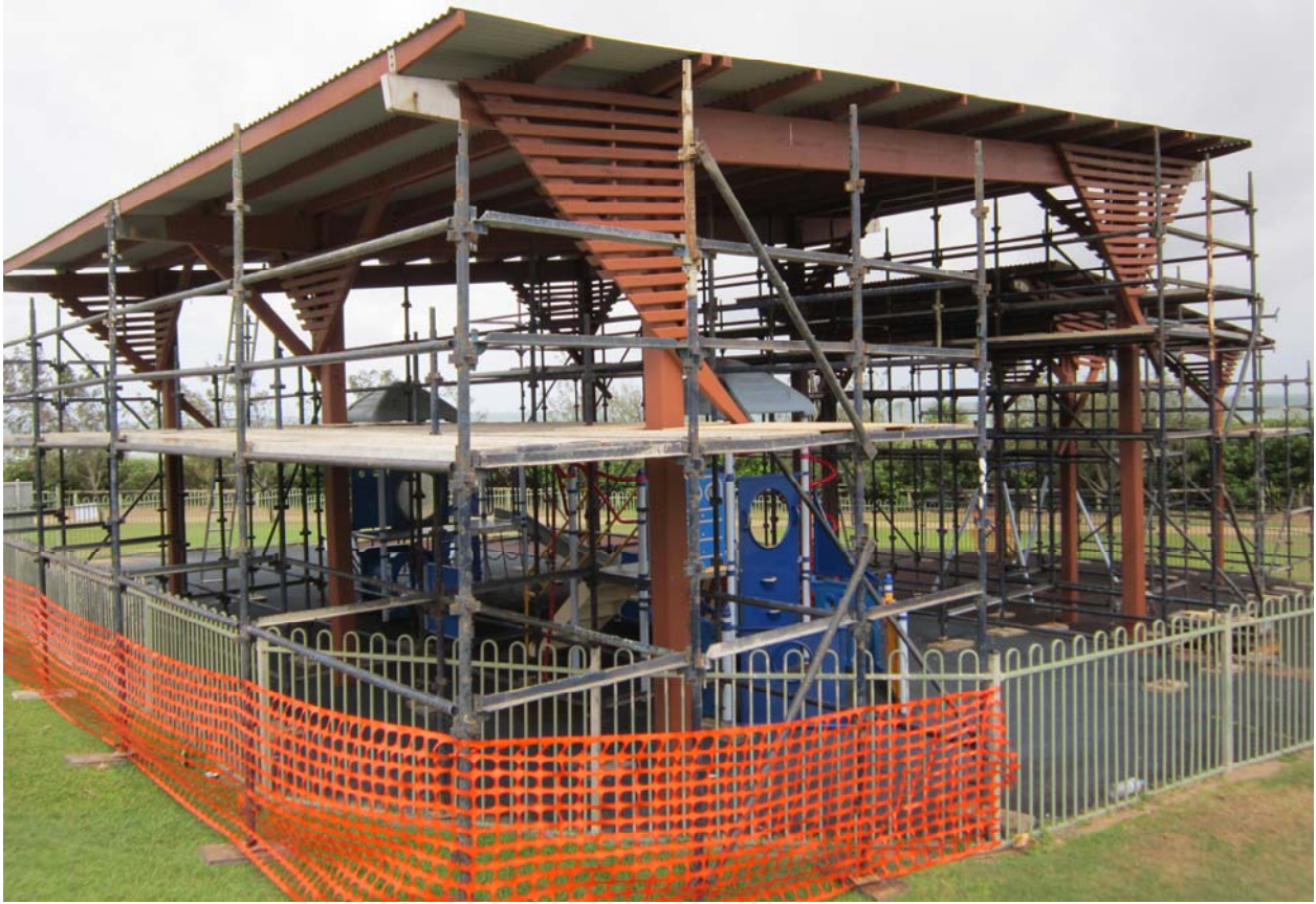
Repairs, Tensioning of bolts and fixings and full repaint, Mulherin Park Shelter
