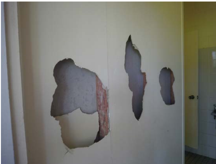
Queens Park Vandalism
