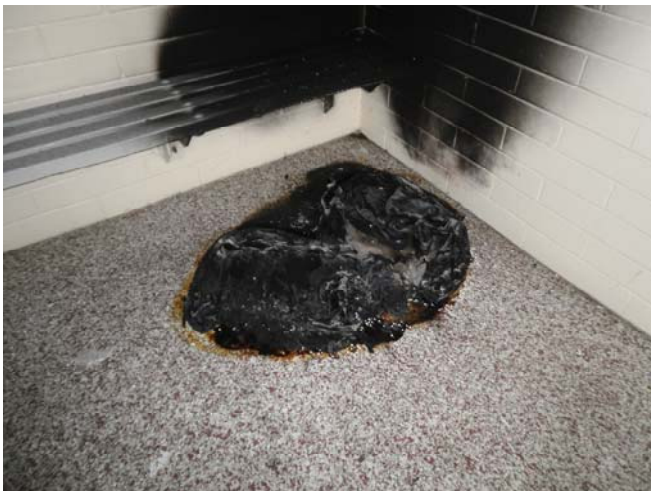
John Breen Park Fire Damage
