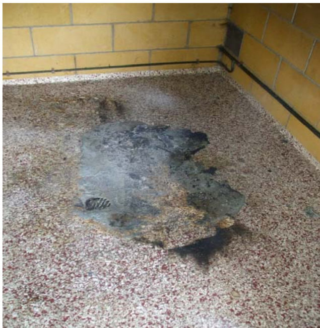
Fire Damage Anzac Park
