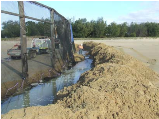
The Mackay Beach team repaired the swimming enclosure at Bucasia, including reburying the net weights
