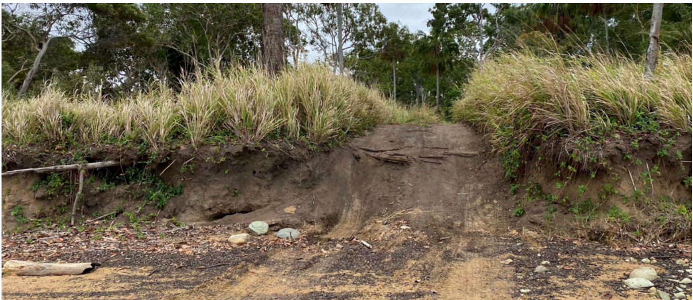
Figure 35: Tyre tracks on Johnsons Beach (top). Informal access track through the dunes and localised erosion scarps (bottom).
