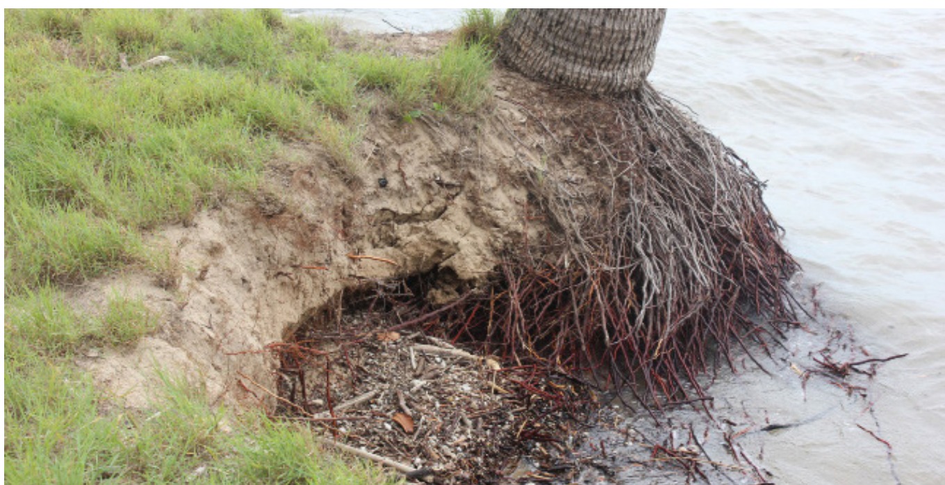
Figure 18: Coconut palms do little to stabilise dune sediment from erosion. It is evident from these pictures taken at McEwens Beach that the confined root-ball is stabilising only a very limited area of dune. More extensive and far-reaching root systems, such as those from coastal she-oaks, would stabilise a larger area of dune.
