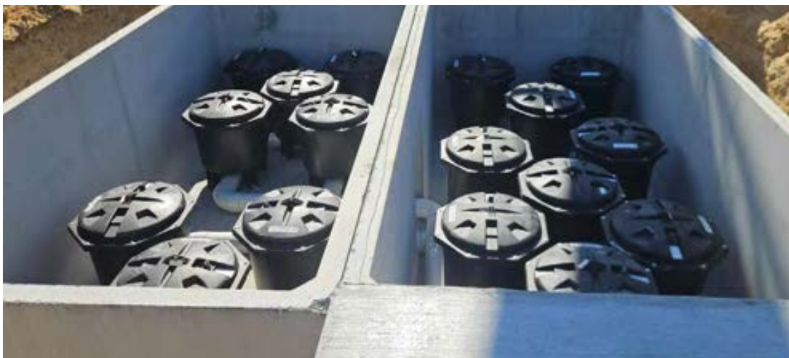
Figure 1 - AtlanFilters in a concrete chamber / vault
