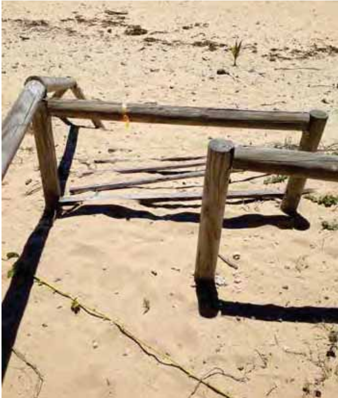
Figure 43: North Harbour Beach access points (SPR01 and SPR02 featured) require remediation.
