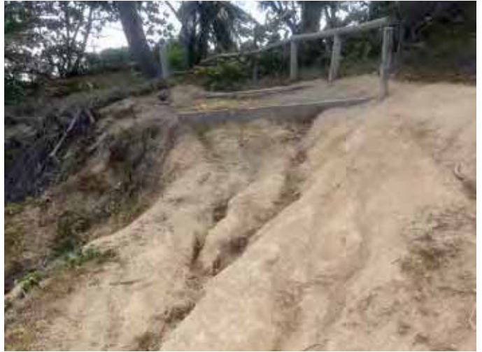
Figure 41a: SLA01, one of two beach access points undermined by erosion.
